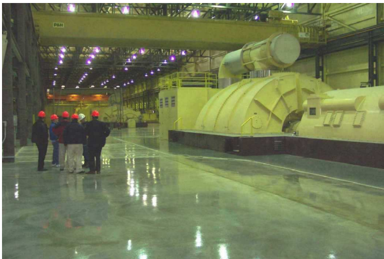
Left -- Tour participants paused to see one of the large electrical turbine generators from which the Spurlock station feeds power to member electric cooperatives throughout Kentucky. Tour participants included Doug Scott, Chad Rausch, Tim Matchett, Bonnie Spencer, Mark Cade, Dan Longpre, Andrea Davis, Doug Davis, Jay Adams, John Shewbrooks and Jim Brown.
